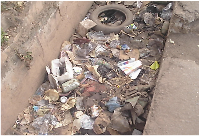
Plate 3: Water Incursion at the Rotary drainage
