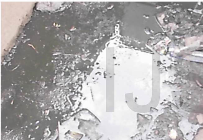
Plate 4: Deteriorated pavement surface at the intersection
